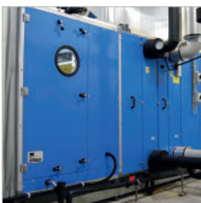
7Air revision front mounted on humidifier section
